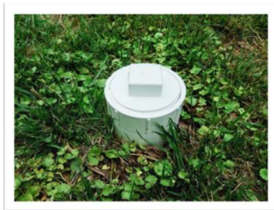
Typical sewer cleanout, 4-inch diameter
